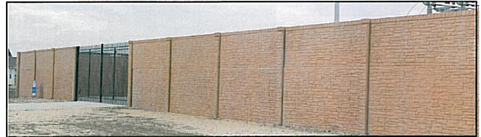
Electrical Substation, Highland, IL
